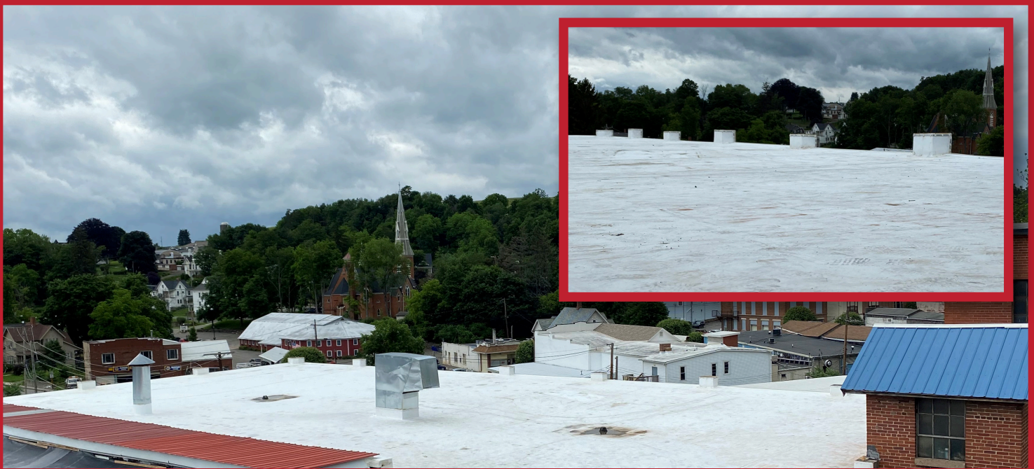
The new white roof coating is designed to help reduce temperatures in the machine shop during the summer months.
